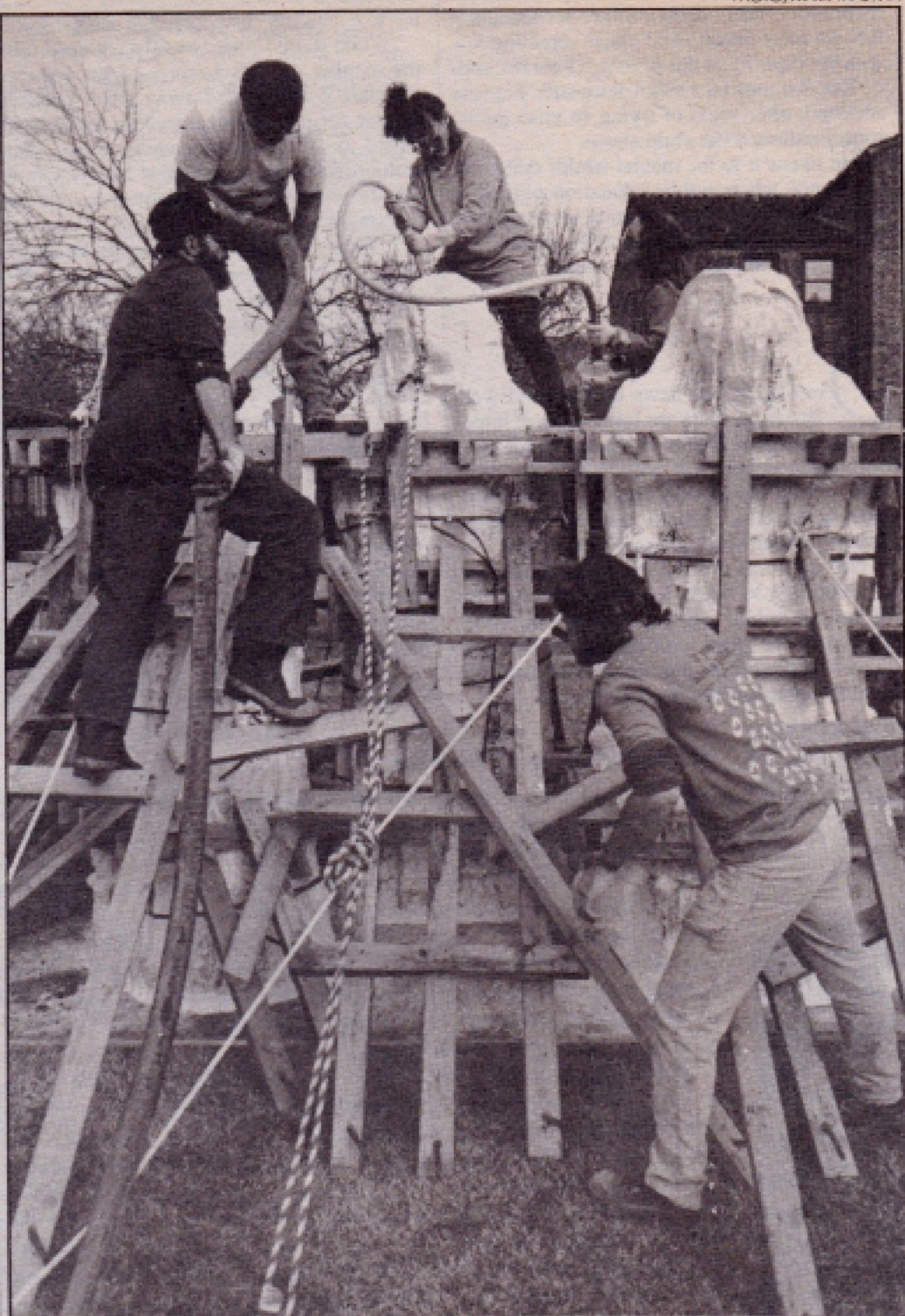
Monolithic Sculpture: Three more monolith structures are being erected on the Chico State University campus. The project is being led by visiting art professor Deborah Masters, pictured at the top on the structures, at right. Masters is using a vibrator to compress the concrete for the eight-foot-high sculptures, while assistants supply a steady flow of concrete and help support the sculptures. The sculptures are located near the campus rose garden.
